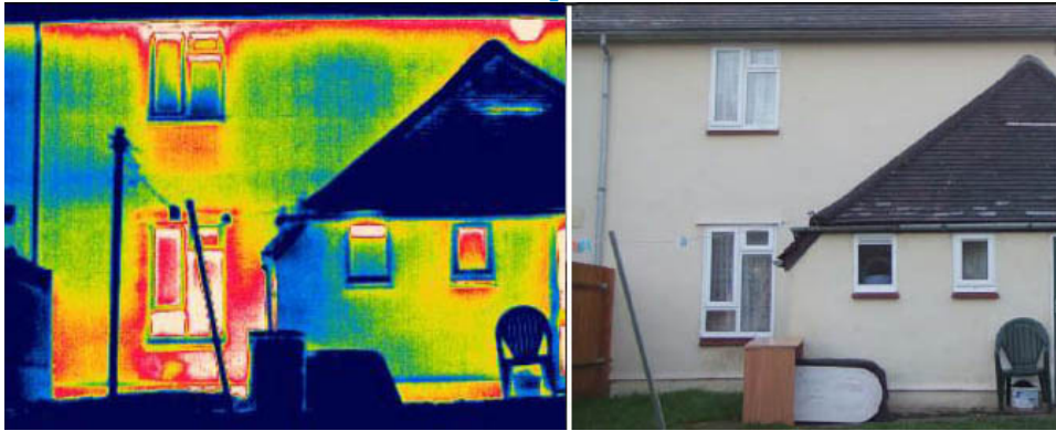
Solid wall dwelling losing significant heat identified by Thermal Inspections Ltd for Dacorum Borough Council
